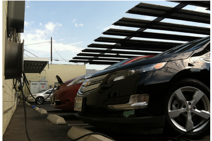
Re-charging in CALSTART's Parking lot
