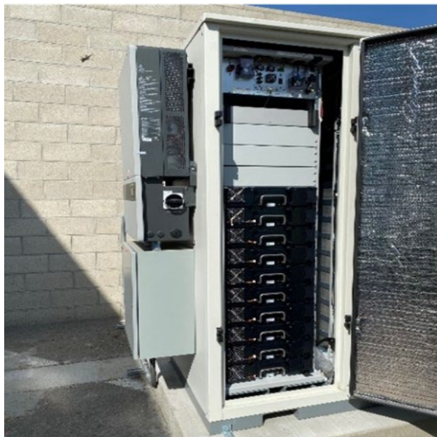
Figure 23: Battery Storage System at DHE
